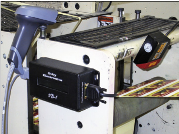
Pre installation ORBY VB1 with hand held and fixed mount scanner.
